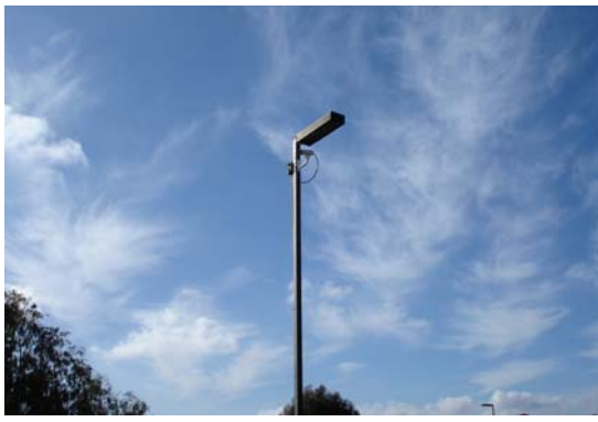
Figure 5. A photograph of the high-performance Sony XCD-X710CR video camera installed on a light post located at the western abutment of the Voigt Bridge. The video monitoring system records bridge traffic continuously and stores data at a centralized data repository (Fraser et al. 2006).
