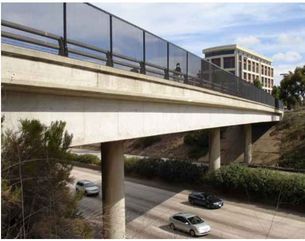
Figure 1. A photograph of the Voigt Bridge crossing Interstate 5 taken from the western abutment. The bridge itself experiences low levels of vehicle and pedestrian traffic during the experimental phase of this study.
